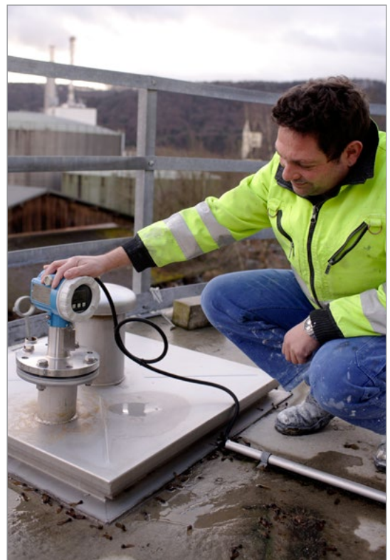
Level instruments are often placed on the lids of storage tanks.
