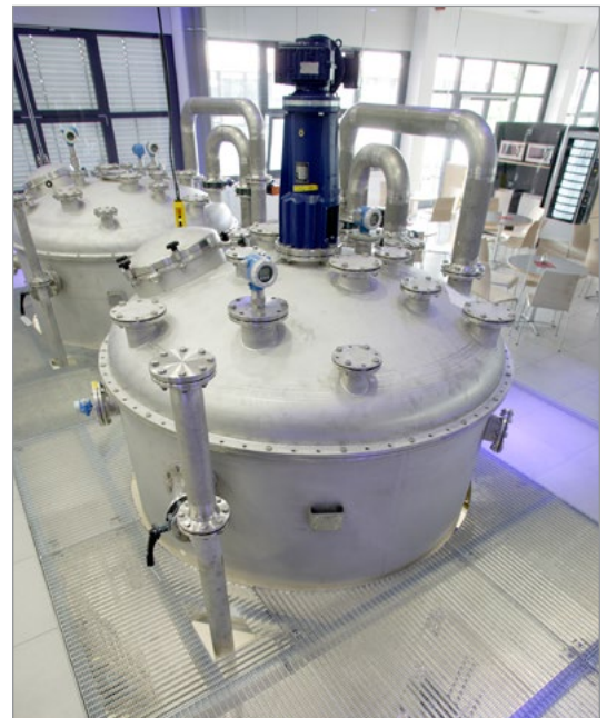
A tank facility at the test center in Maulburg.
